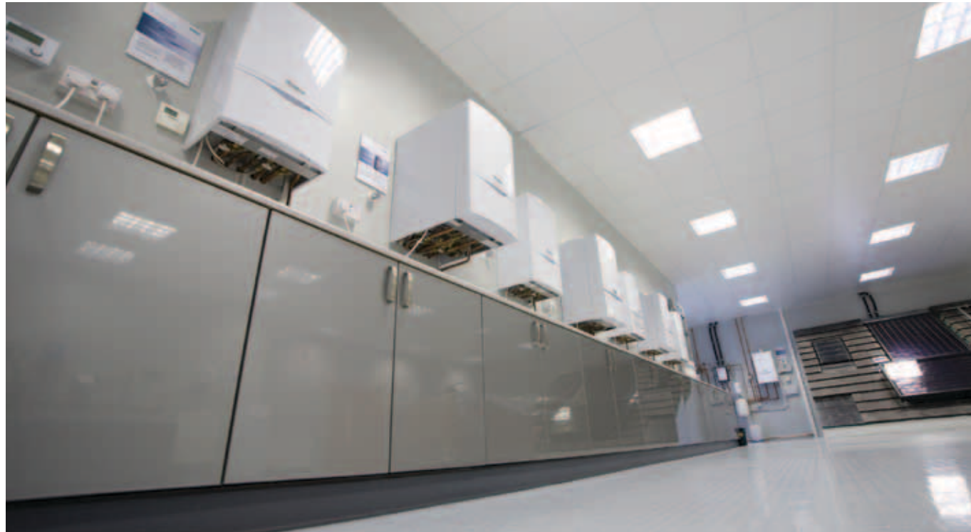
State of the art Vaillant Training Centre in Bristol
