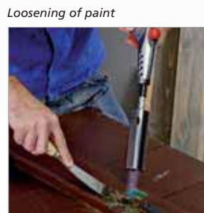
Loosening of paint
