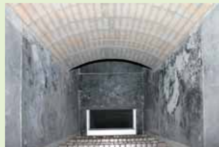
Fully ceramic-lined combustion chamber with air-cooled grate
